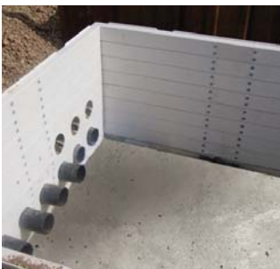
Multiple duct lines
